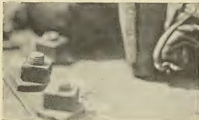
Fig. 17.—Rivet in Center Foreground Partially Driven, Showing That Rivet is Driven Straight Down With Concave Set to Swell Shank and Completely Fill Hole. Metal Expanded Equally in All Directions. Rivet is Still to Be Driven Securely Into Countersink, Calked and Excess Material Removed
